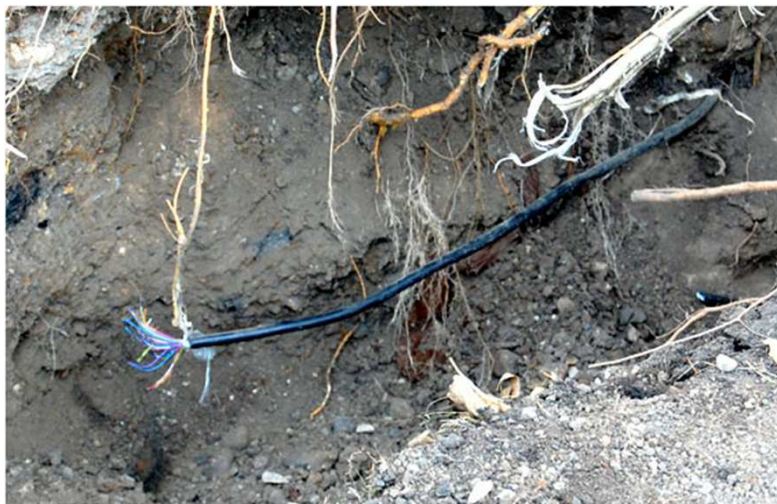
Cut cable (electrical open)
